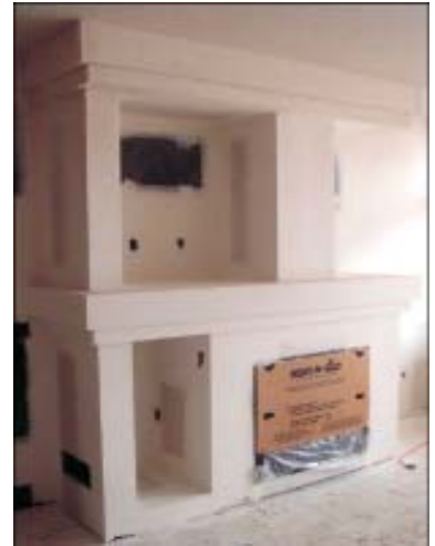
Right, a completed unit ready to receive zero clearance fireplace, TV set and stereo.
